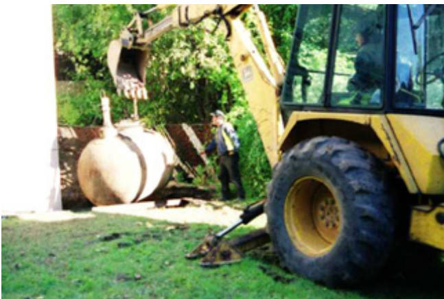
Removal of an Underground Storage Tank (UST) to prevent future groundwater pollution.
