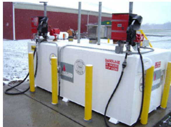
Fuel dispensing system with secondary containment at Snyder Farm.
